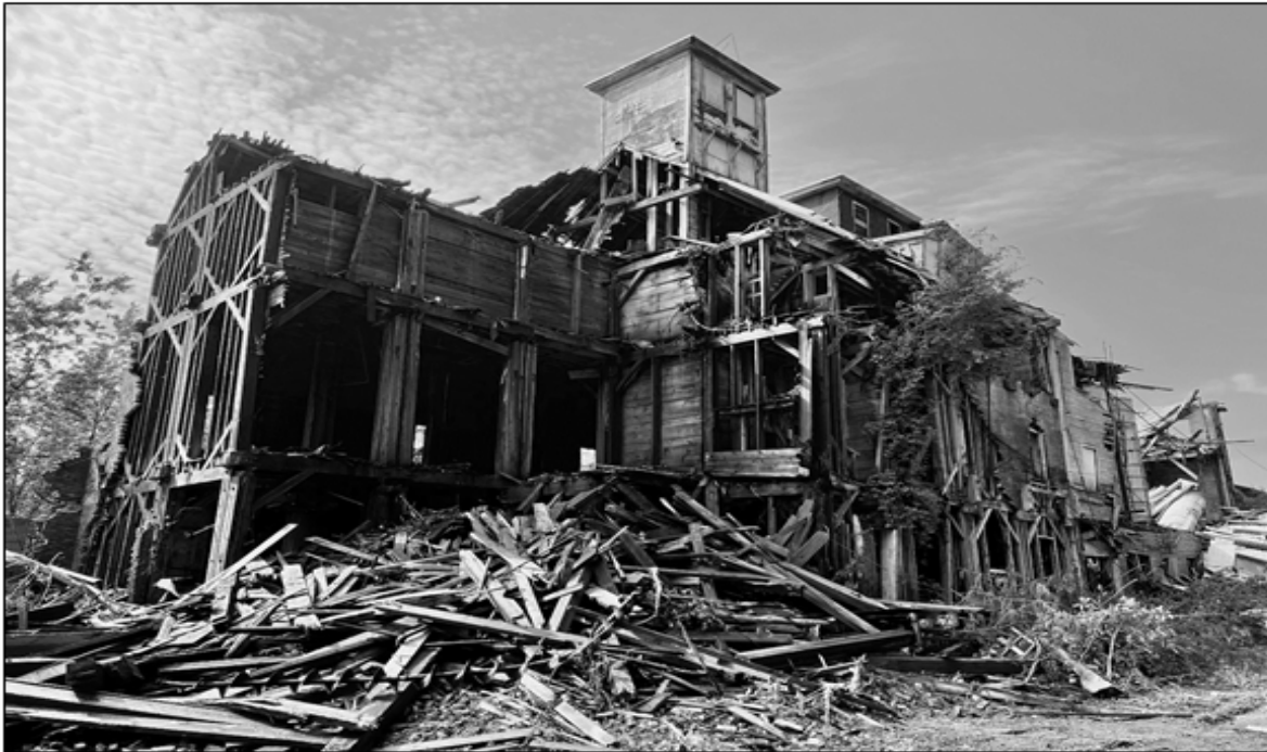
The Town-owned Commercial Street buildings just prior to demolition in the fall of 2022.
