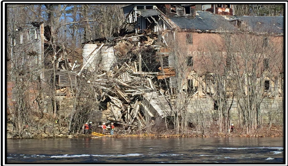
View across the river from the Hannah Dustin Island. How many demolition workers can you find?
