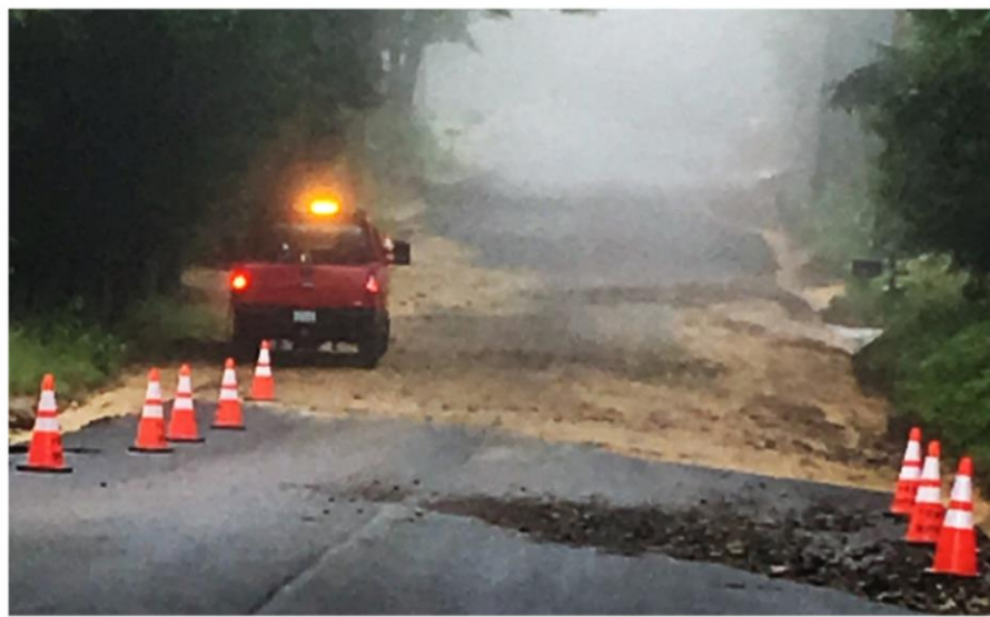
Goodhue Road Washout after Paving, Severe Storm & Flood of October 2017 Photo courtesy of: Public Works Department
