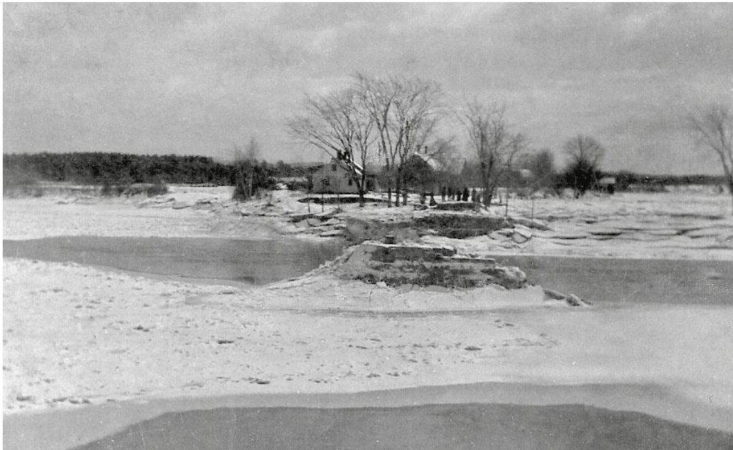
View of the bridge abutments facing Concord after flood
