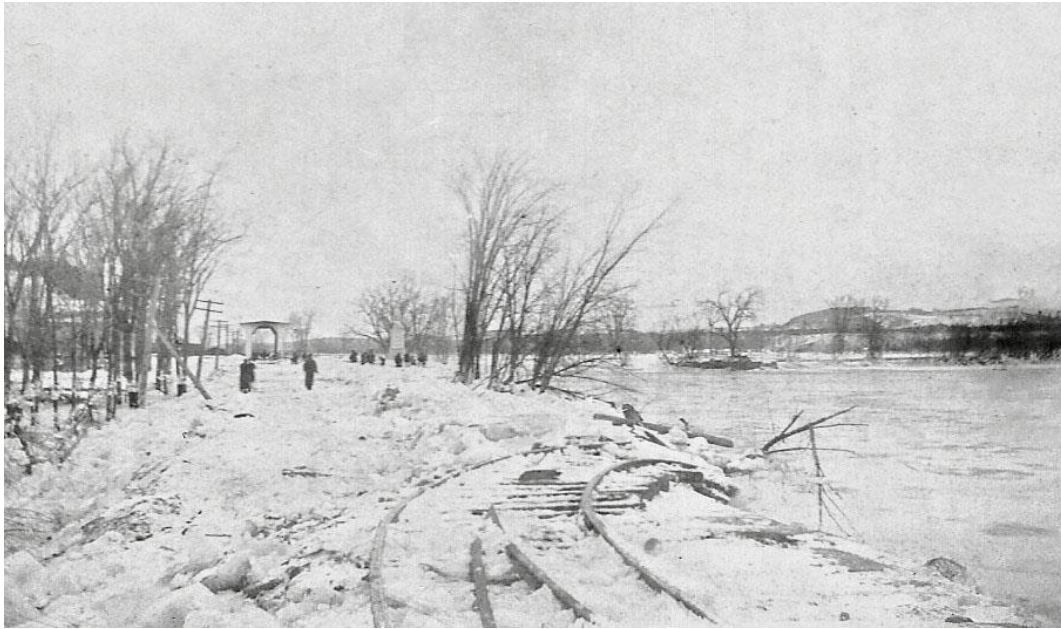
Damage to the railroad tracks with the Hannah Dustin Island in the background
