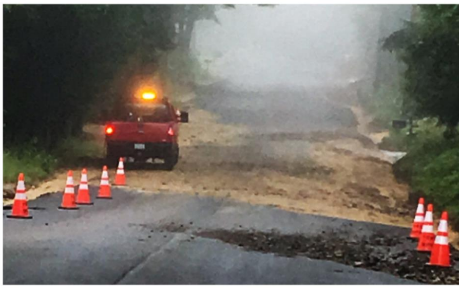
Goodhue Road Washout after Paving, Severe Storm & Flood of October 2017 Photo courtesy of: Public Works Department
