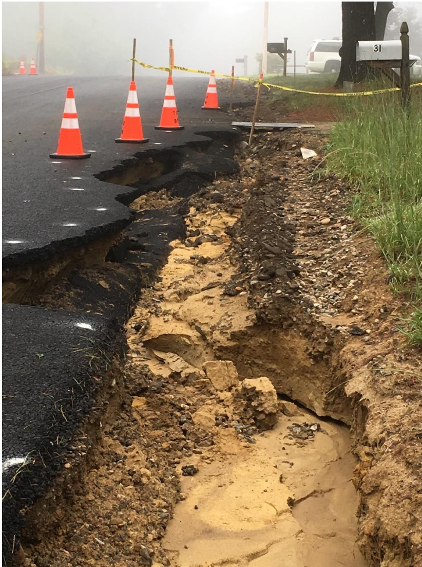
Goodhue Road Washout from October 2017 Storms
