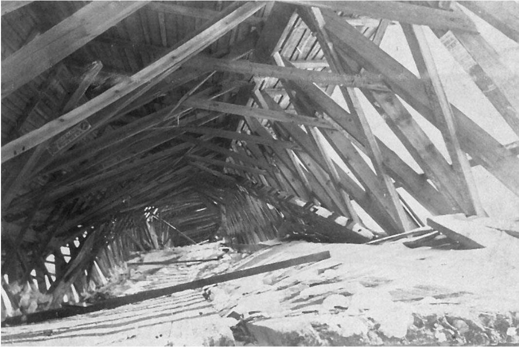
Boscawen-Concord Bridge View of the damaged bridge from the inside
