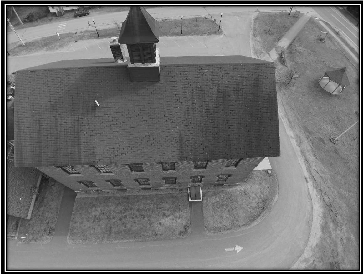
Mike Bradford took this picture with his drone to inspect the shingles on the roof of the Municipal Complex.
